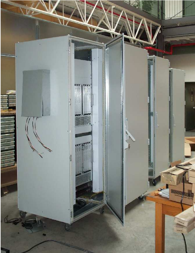
The ACSIS enclosures in the lab area at DRAO. The enclosure on the left has been fitted with two of the correlator crates.
