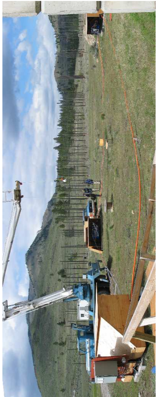
The winch test described in the text. The “cherry-picker” truck tensions the tethers. The conduit running into and out of the winch enclosures contains the optical fibre used for communications.
